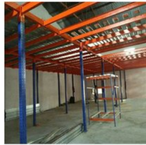
Modular Mezzanine Floor
